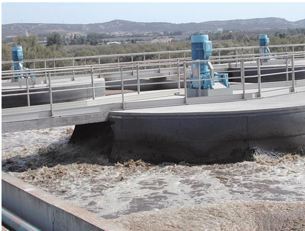
Figure 15 : Basin for biological treatment of wastewater with surface aerator (Photo: courtesy of Socié'té des Eaux de Marseille)
