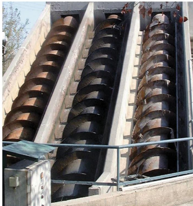
Figure 12 : Screw lift (treatment plant of the town of Vitrolles, France) (Photo: courtesy of Societe des Eaux de Marseille)
