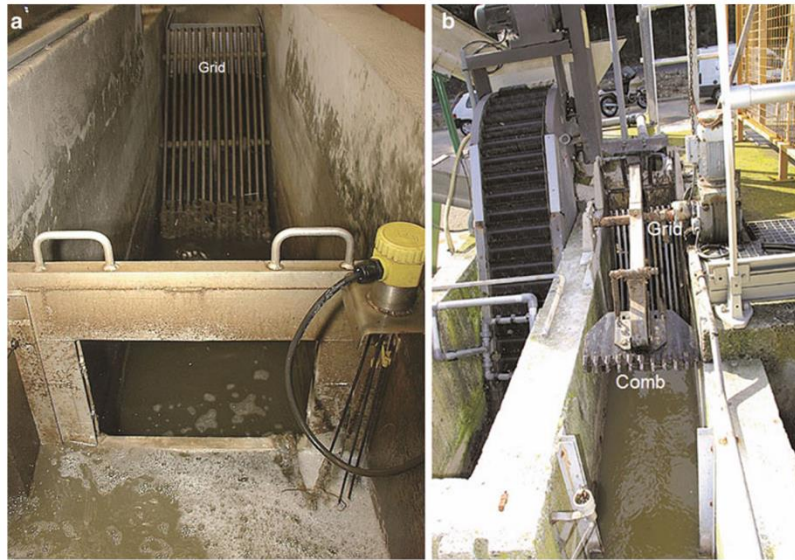
Figure 11 : Example of screening. (a) Grid screening; (b): grid and comb for elimination of accumulated pollution on the grid (Photographs courtesy of Societe des Eaux de Marseille)
